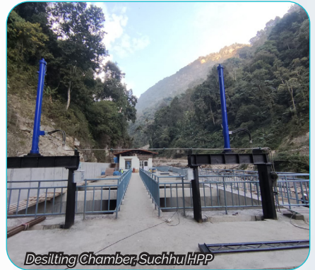
Desilting Chamber, Suchhu HPP
